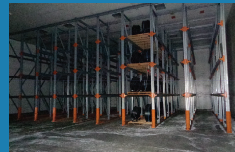
Drive Thru racking
