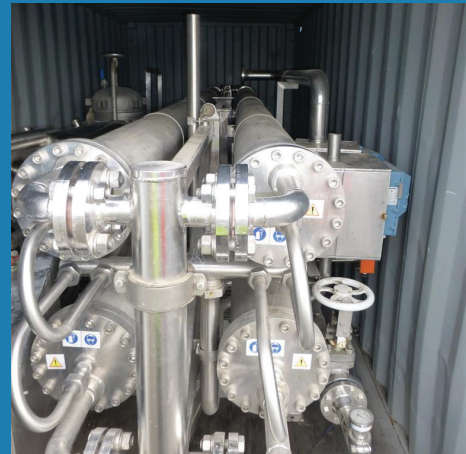
Reverse Osmosis Plant
