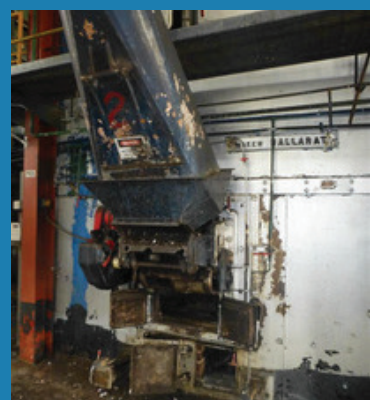
Babcock Coal Boiler
