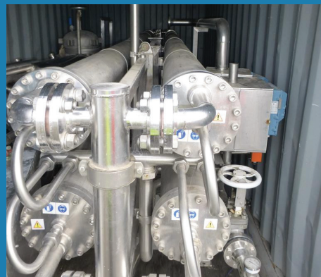
Ultra Filtration Plant
